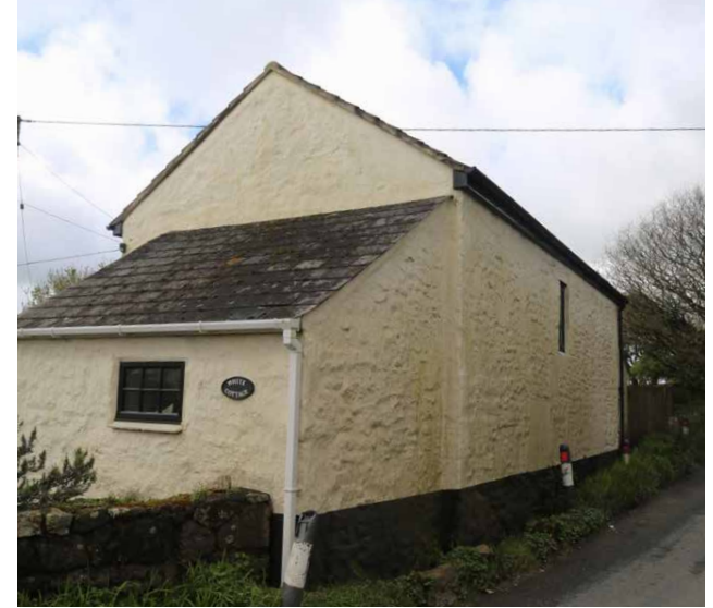
Figure 45: Rubble stone texture behind lime wash façade .
