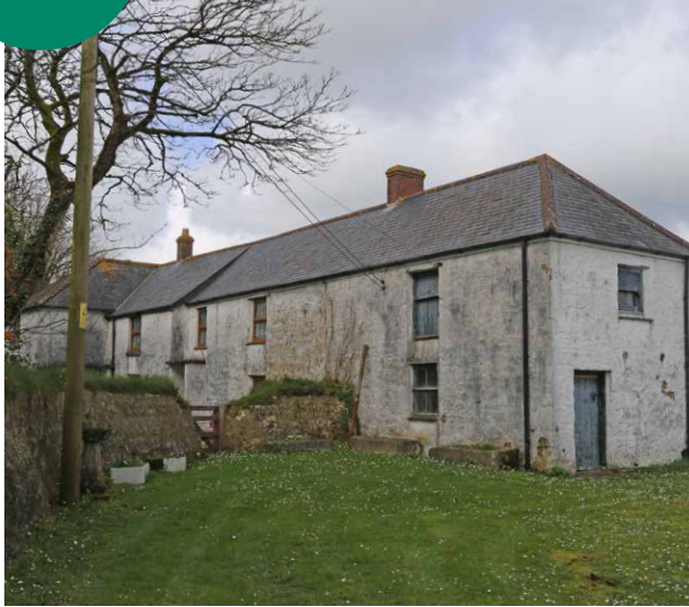
Figure 14: Tall well-proportioned farmhouse albeit in disrepair, in crosswing arrangement with hipped roof and brick chimneys.
